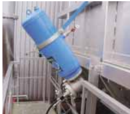
Recycling plant Glasses powder silo
