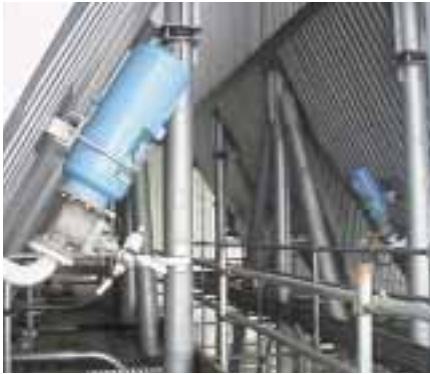
Incinerator plant Incinerator ash silo
