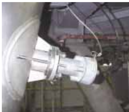
Petrochemical plant Storage tank Plastics pellet
